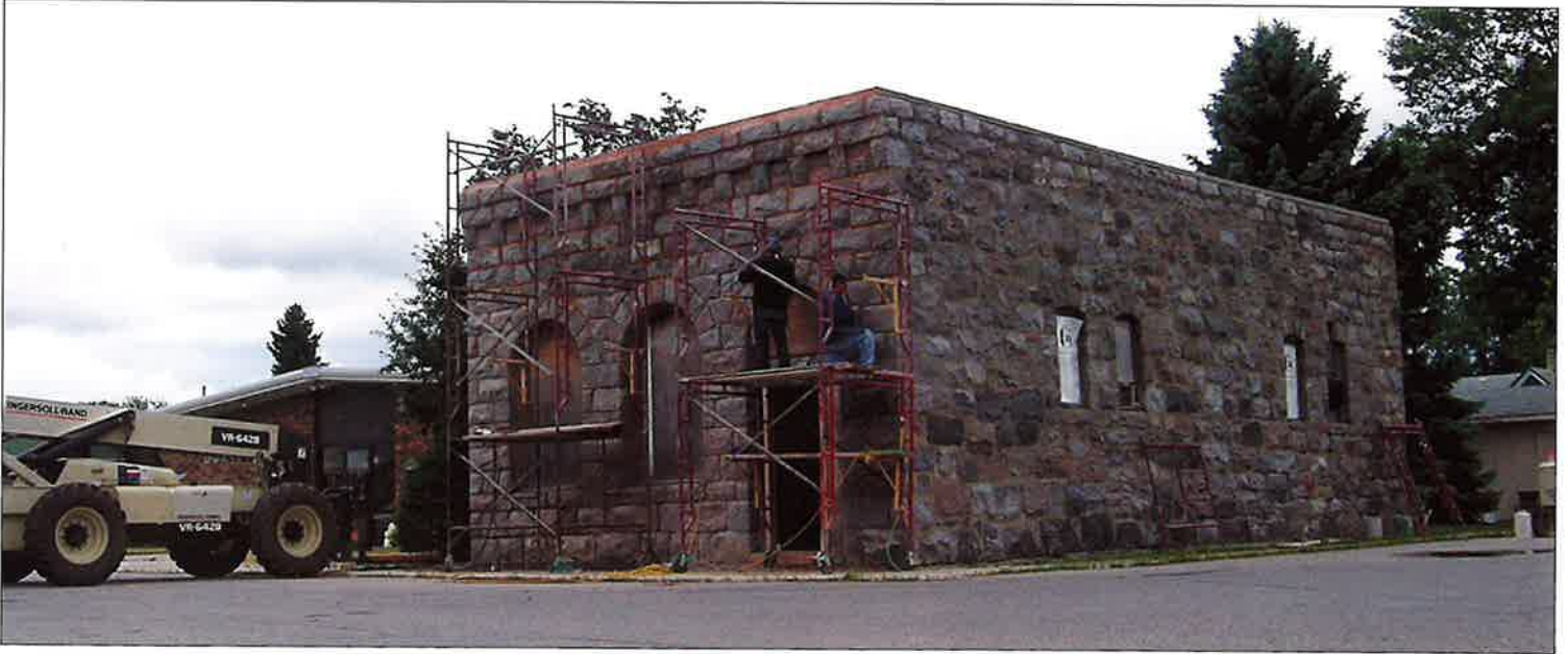
Above: Larry Schornack and Marlin Lenior of Nelson Masonry, Grand Forks, set up scaffolding to repair the mortar joints between the stone, a process called tuckpointing. Below: Nelson Masonry's Dave Reuther (left) and Larry Schornack repair mortar joints on the north side of the bank.
